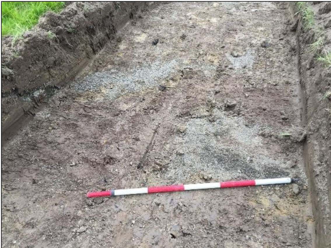
Plate 14: Pea gravel indicating buried underground services towards the northeast end of Trench 3
